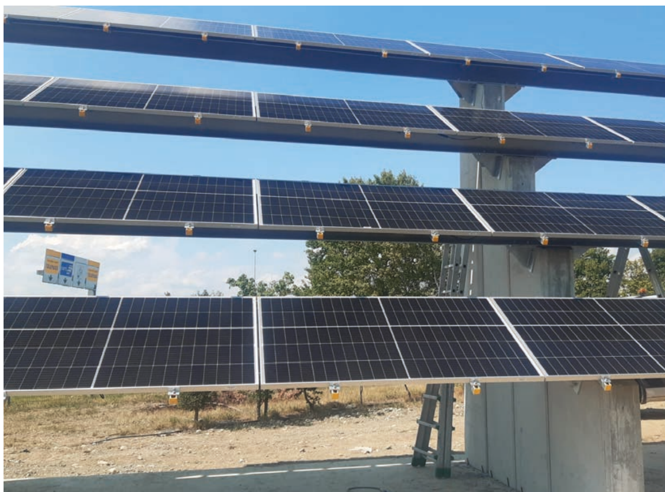
S.A.T.A.P S.P.A. - Photovoltaic Plant, Biandrate
