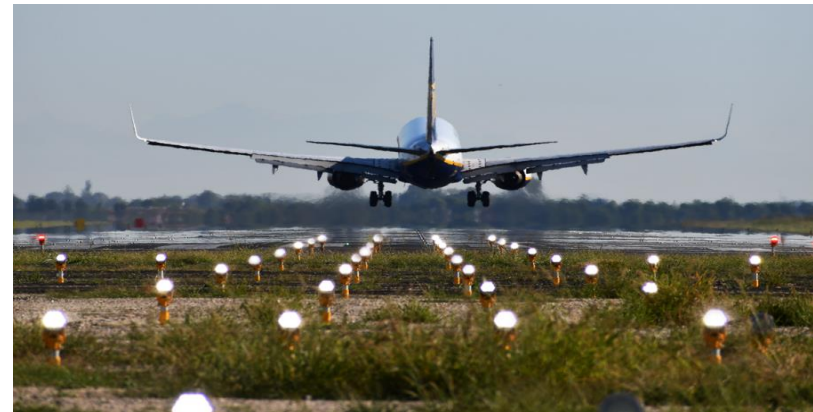
Client: SAVE S.P.A. Description: Implementation of special installations in airside area, specifically electrical and mechanical installations for the airport of Venice
