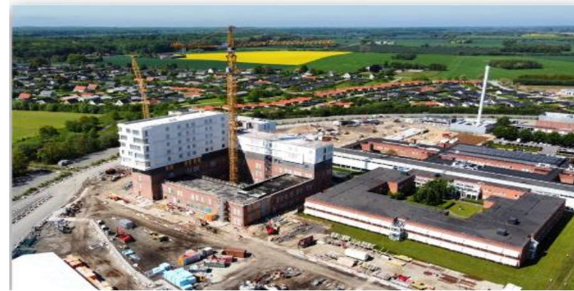
Client: KOGE HOSPITAL PROJECT TEAM I/S Description: Implementation of all works pertaining to the electromechanical part of Zeeland University Hospital in Køge, Denmark
