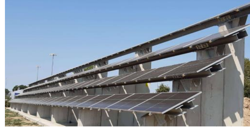
Client: S.A.T.A.P.S.P.A. Description: Photovoltaic System Biandrate
