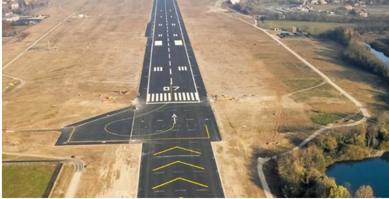
Client: SAVE S.P.A. Description: Rehabilitation runways, apron and hangar construction Marco Polo Airport - Venice - Tessera
